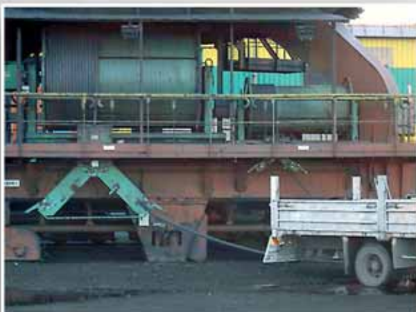
Iron Ore Scrapper. Power and control level wind reels driven by permanent magnet couplers.
