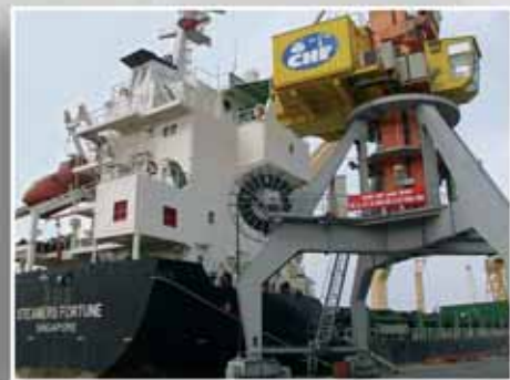
Power cable reel on a mobile swiveling ship unloader.
